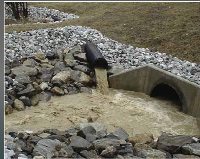
Photo courtesy of WNY Stormwater Coalition.
