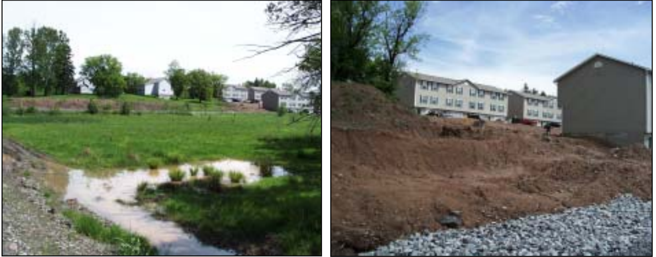
Figure 10. Construction at site 10b showing exposed soil on a steep embankment and proximity of creek, 25 May 2004.
