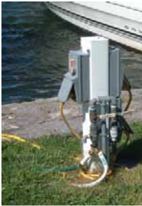
Water and electric service facility for boats.
