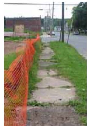
A Village sidewalk in need of repair.
